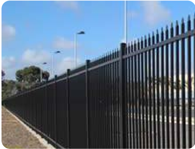
Boundary Fencing (1.8m Black Palisade Fence)
